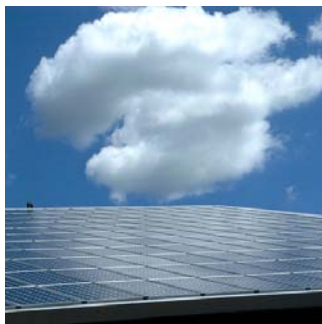
Photovoltaic panels with Arkema polymers.
